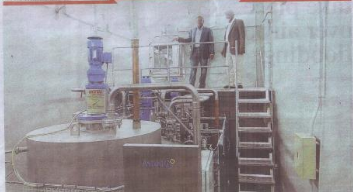
VETERINARY RESEARCH FACILITY HAS AN ANIMAL ROOM AT THE RM32 MILLION RESEARCH FACILITY IN JERU. PIC BY MAHMOUD HASSAN
